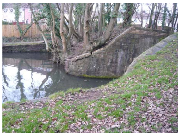
Deteriorating Condition of the lock wing wall
