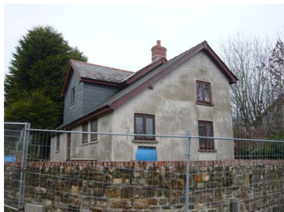
The former Lock Keepers Cottage, delisted due to inappropriate alterations
