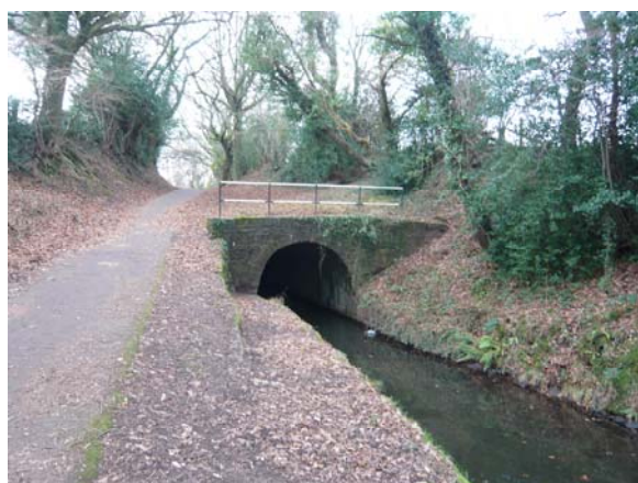
The northern end of the listed and only tunnel along the Torfaen section of the Canal
