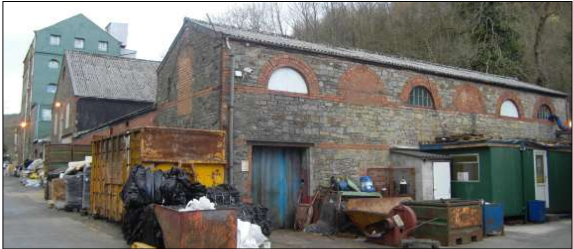
Rear industrial buildings requiring maintenance and appropriate repairs
