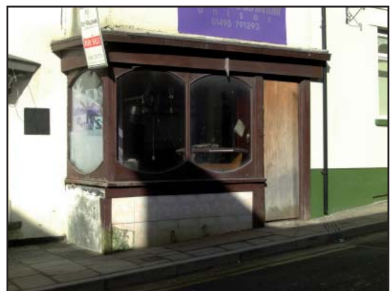
Poor quality, inappropriate designs and / or badly maintained or derelict shop fronts have a detrimental impact on the street scene and the economic health of the area.
