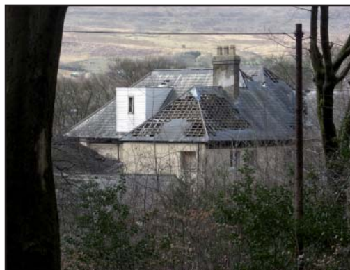
Dormers on heritage properties should ideally be removed where their scale, form, materials and / or proportions are not in keeping with the original building.
