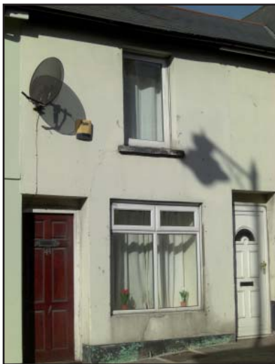
Changes to the proportions and size of window openings has a major impact on the balance of the building, particularly in a terrace where it is the repetition and uniformity of the elevational treatment which gives it its character.
