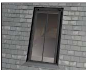
Where rooflights are being incorporated, consideration should be given to using a conservation-type design with a vertical glazing bar as illustrated here.
