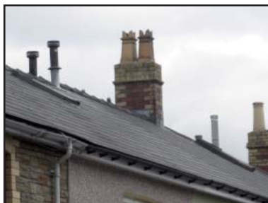
Where chimney stacks have been removed, ugly boiler flues are sometimes still required, giving additional need for the retention or reinstatement of the original structure.
