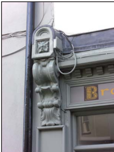
Cables and other fixtures on the exterior of buildings need to be avoided if possible and, at the very least, carefully located and fixed.
