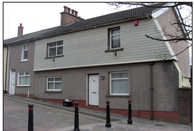
Putting a cladding material on top of the original structure is not appropriate within the conservation area or for heritage buildings within the WHS. Here, the windows and doors are also out of keeping with the heritage character.
