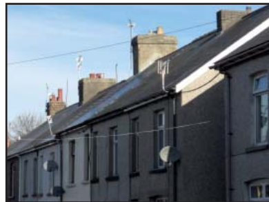
Where chimney pots have been removed the roof profile loses an important part of its consistency and regularity of rhythm.
