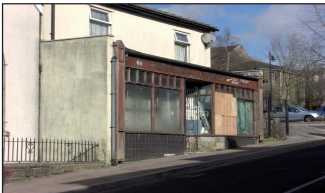
Buildings in a poor state of repair have a detrimental impact on the wider area.
