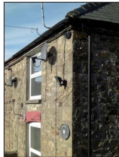
Aerials, lighting, satellite dishes and electrical fixtures all contribute to diminish the simple uncluttered qualities of the traditional building form in Blaenavon.
