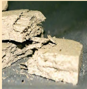
Asbestos Insulating Board.
