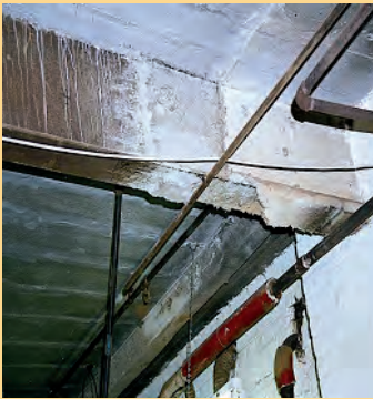
Sprayed Asbestos and Lagging.
