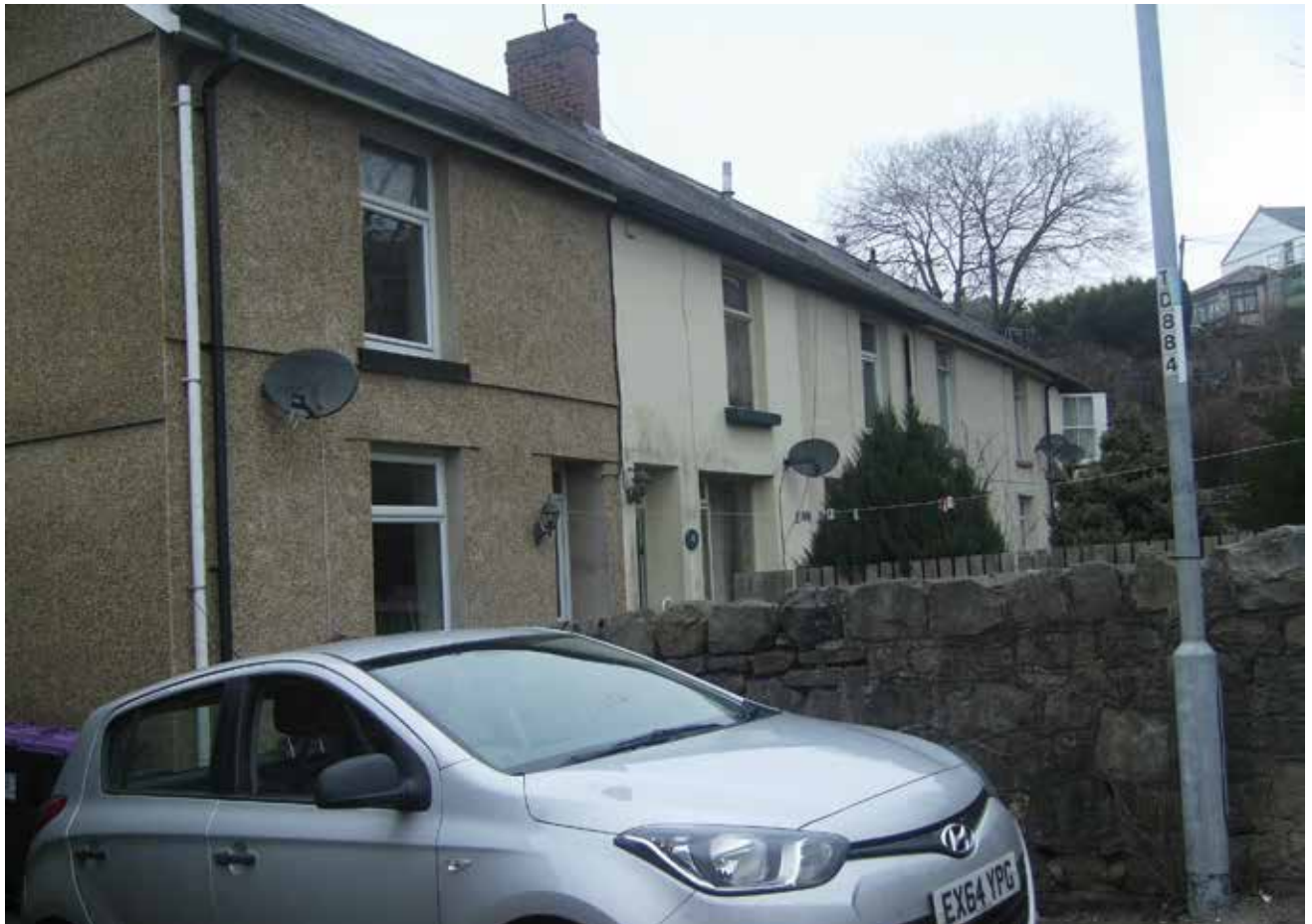
Loss of chimney stacks and pots, windows and doors with inappropriate wall finishes change the character and design of this traditional terrace.
