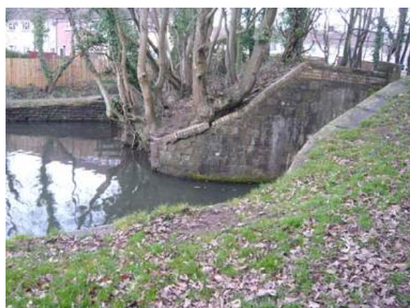
Deteriorating Condition of the lock wing wall
